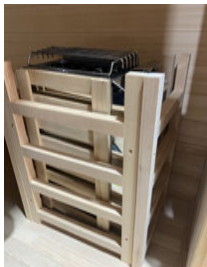
location of the stove
