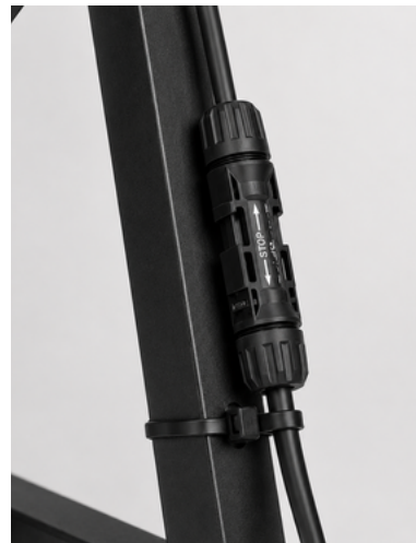
MC4 connection cable secured with a cable tie
